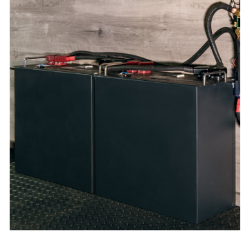
(2) 200AH 24V Lithium Batteries (which is equal to (8) 100AH 12V Lithium Batteries)*
