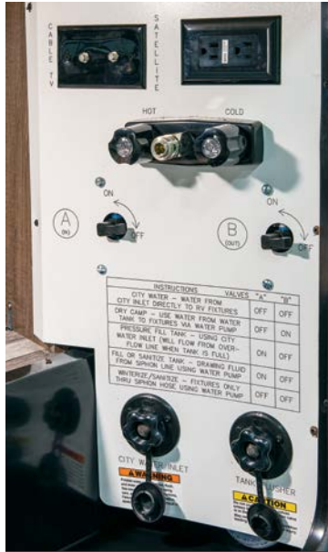
CENTRALIZED COMMAND CENTER heated & all systems conveniently located
