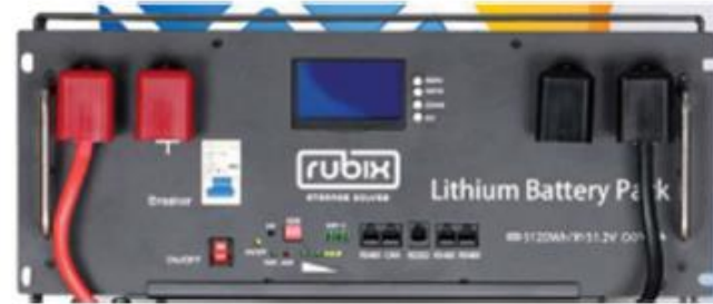
Battery (front view)
